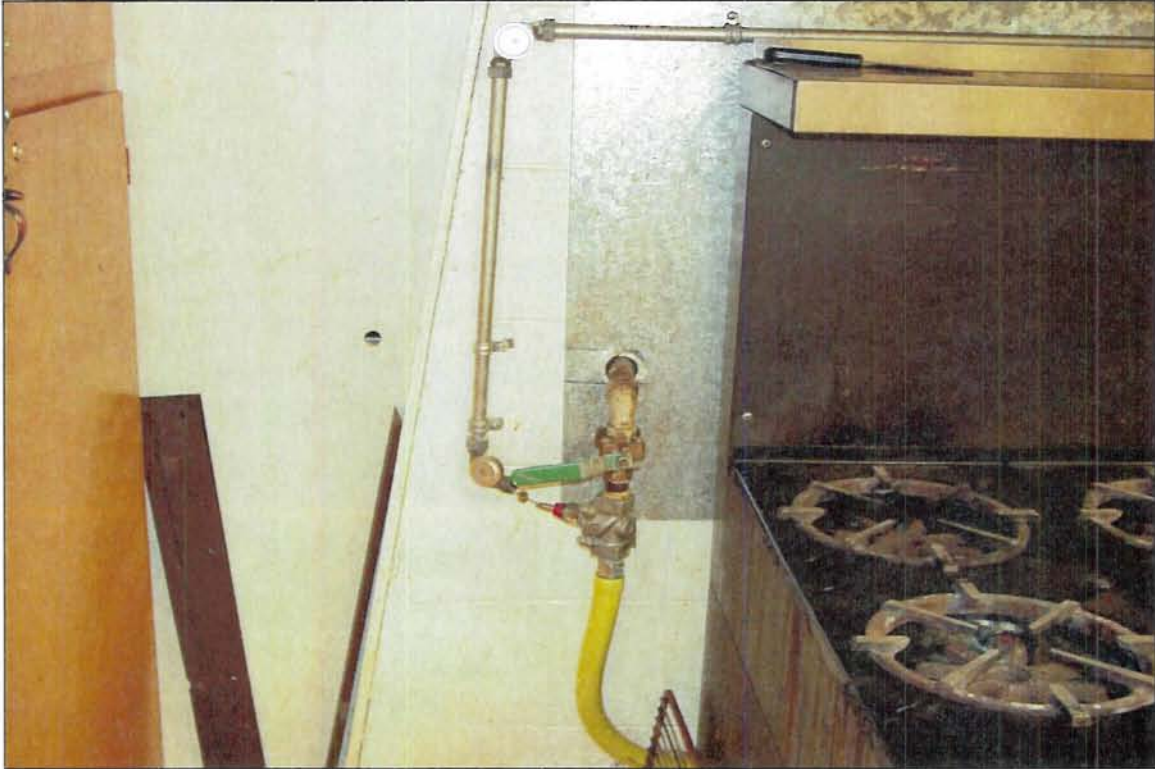
Photo 13 - No Label On Propane Shut Off
