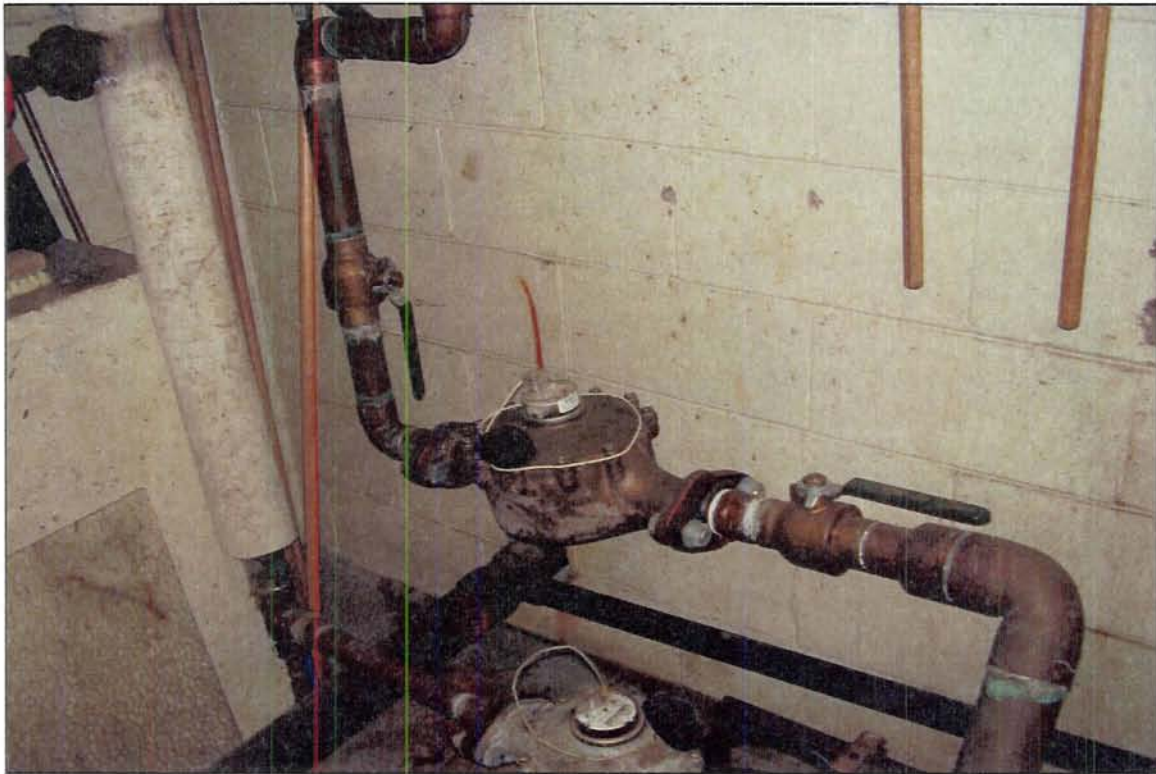
Photo 7 – View of Water Meter and Entrance
