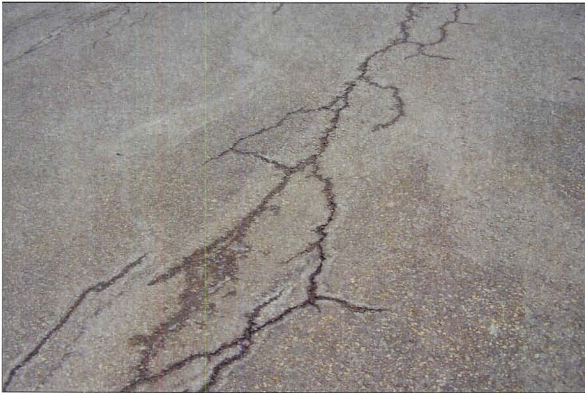
Photo 18 - Alligator Cracking In Asphalt
