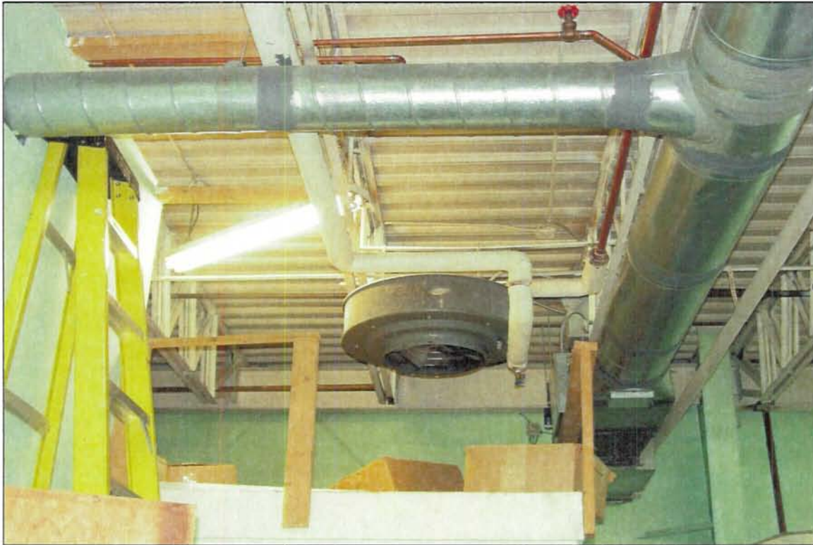
Photo 14 - Unit Heater Over Mezzanine On Main Floor
