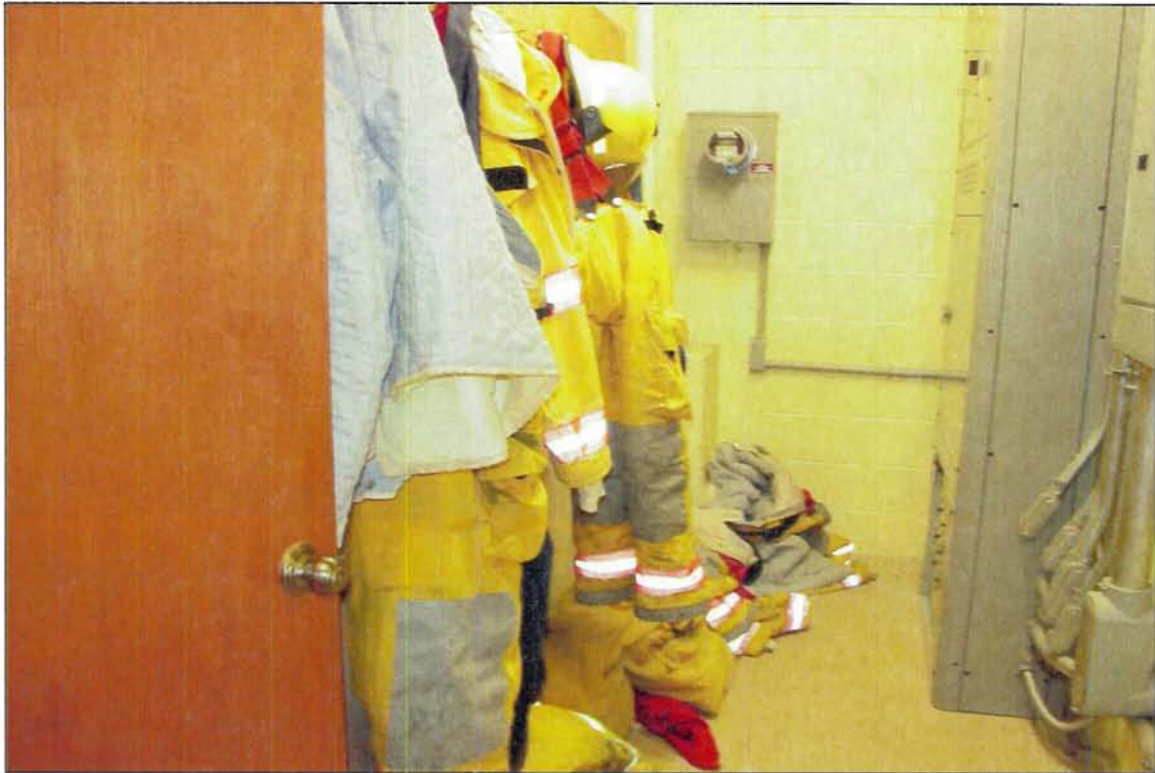
Photo 1 - View Of Electrical Room
