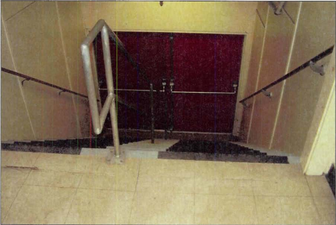
Photo 24 - Non-Compliant Egress Stairs At The Rear Of The Building
