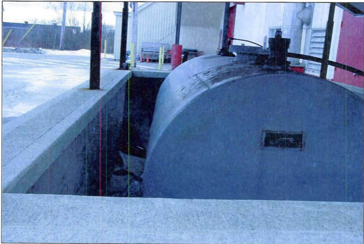
Photo 16 - AST In Concrete Containment. Note Damaged Liner And Ice Buildup
