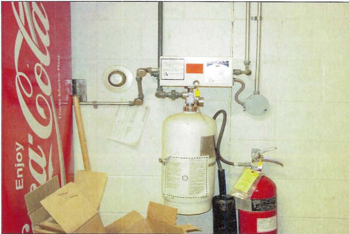
Photo 11 - Manual Activation For Cooktop Fire Suppression System
