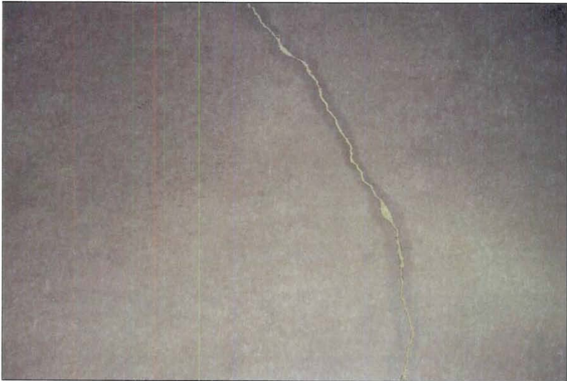
Photo 22 - Cracking In The Concrete Floor Slab
