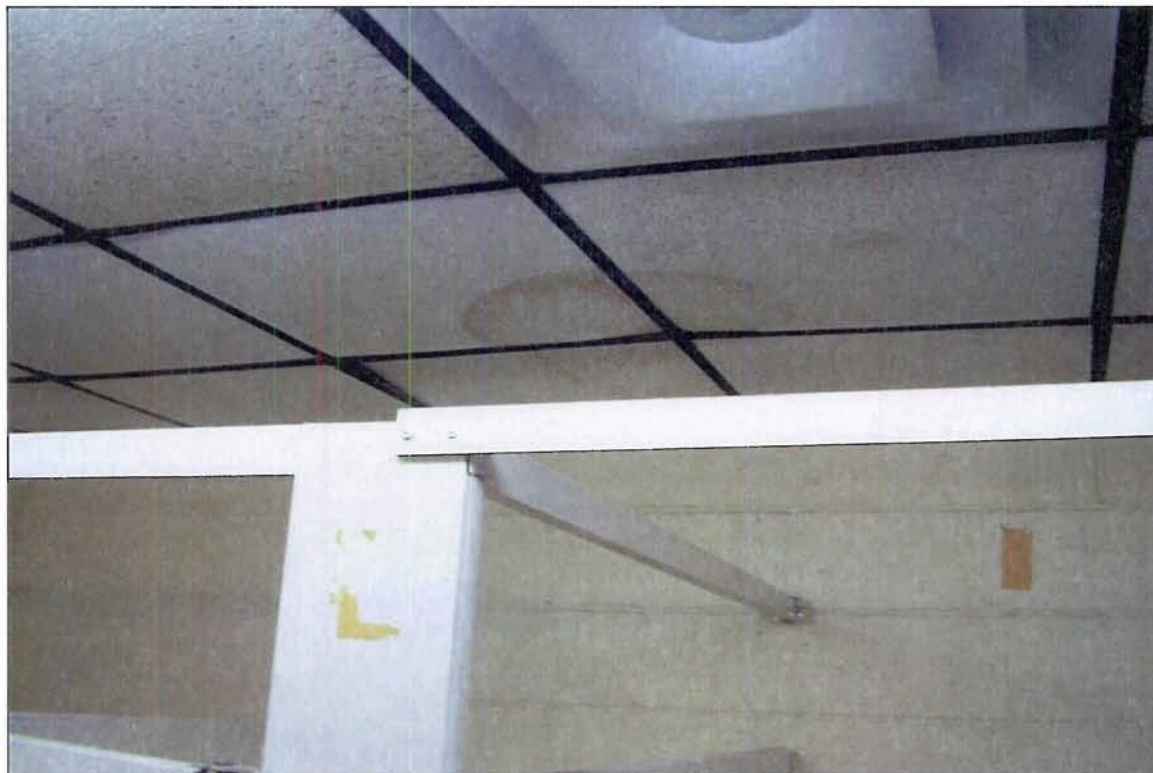
Photo 28 - Stained Ceiling Tile In The Washroom
