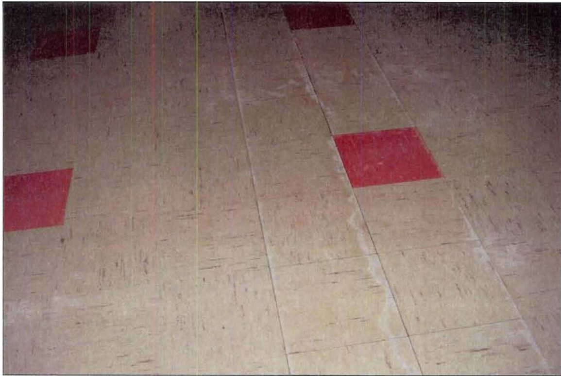
Photo 19 - Cracking In The Second Floor
