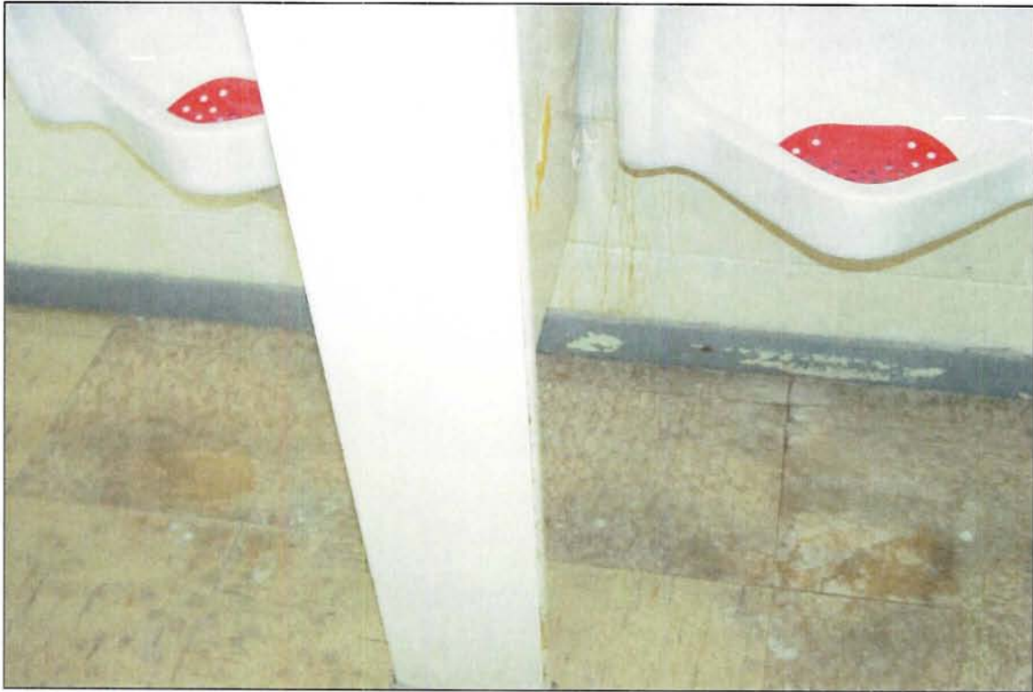
Photo 15 - Evidence Of Past Plumbing Leaks In Main Floor Washroom
